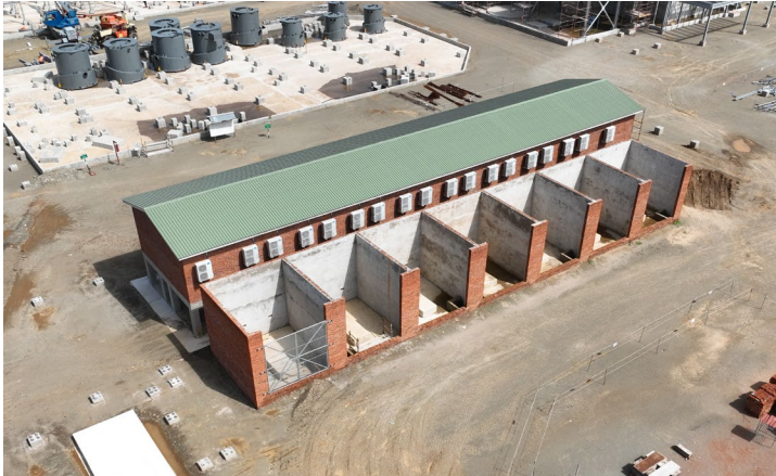
Wet End LV Substation
