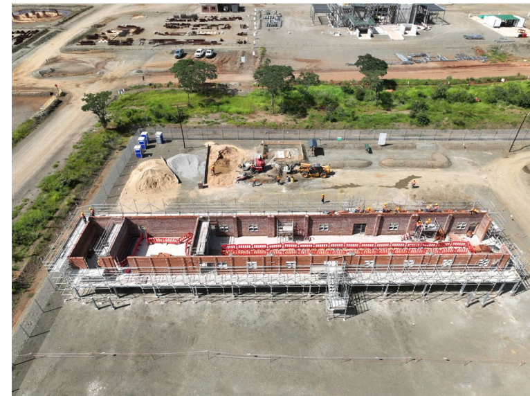
MV Substation Building
